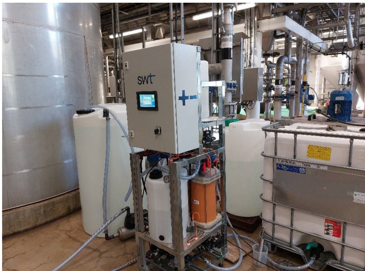
FIGURE 18. The CDI test rig placed in Building B650 at the AstraZeneca Gärtuna site. From the left, the collection tank, CDI unit, reject tank (smaller tank behind the CDI unit) and the test water tank.
